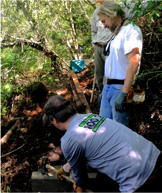
Bob Strayer (above) guides the bridge installation. It took four people to lift the redwood slab and place it across the gully.
