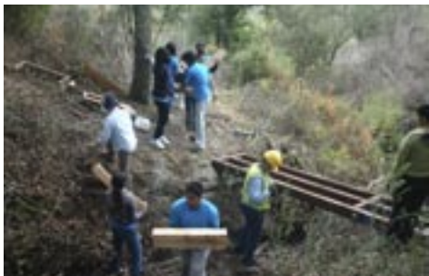
There is something for everyone to do as steps and crossings are assembled.
