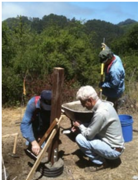
JON KAUFMAN (without cap) helps Tom Klatt secure a new signpost while Lynn Yamashita stirs cement.
